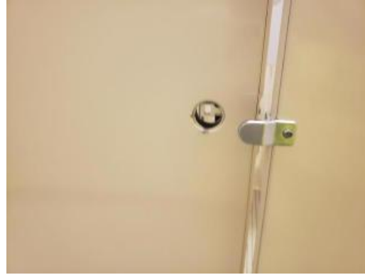
Missing lock on toilet Partition
