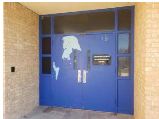
Damaged exterior door
