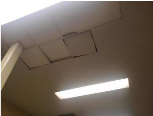
Damaged acoustical ceiling tiles
