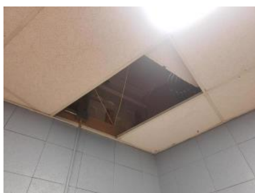
Missing ceiling tiles
