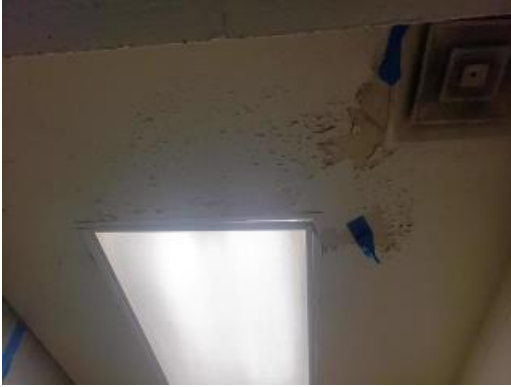
Chipping paint on hard ceiling
