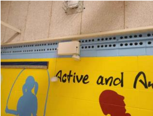
F22 Wall pack emergency lighting is broken
