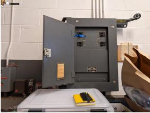
Electrical Distribution Panel at the end of life
