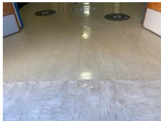
Vinyl composite tile flooring at end of life
