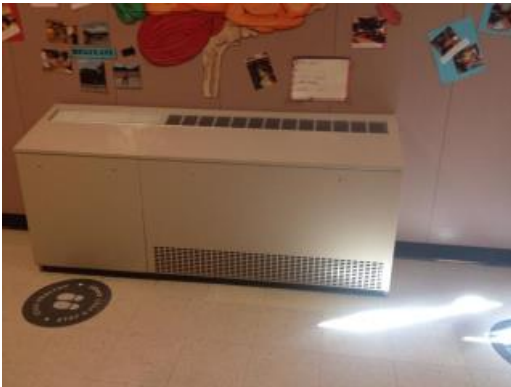
Unit ventilators at end of life
