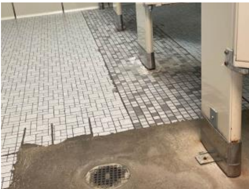
Restroom tile flooring needs finishing or replacement
