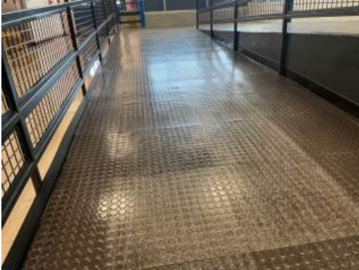
Corridor ADA ramp corners are lifting and numerous tiles are heavily worn
