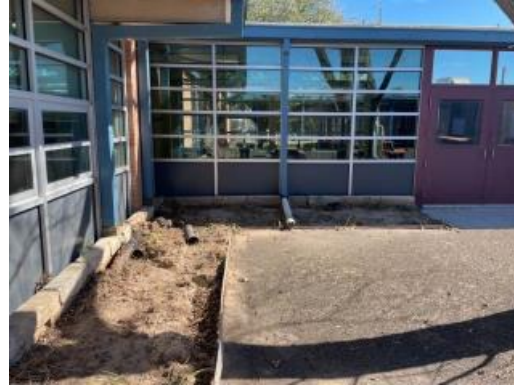
Incomplete grading & drainage for the water intrusion into the hallways
