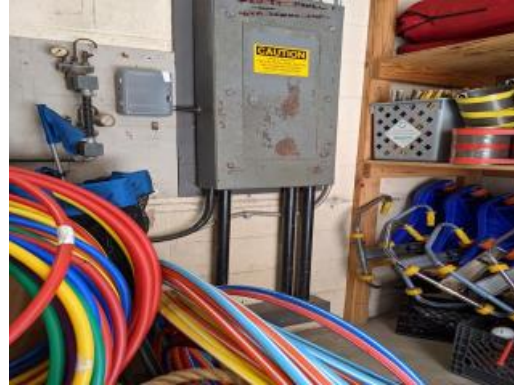
Worn electrical panel
