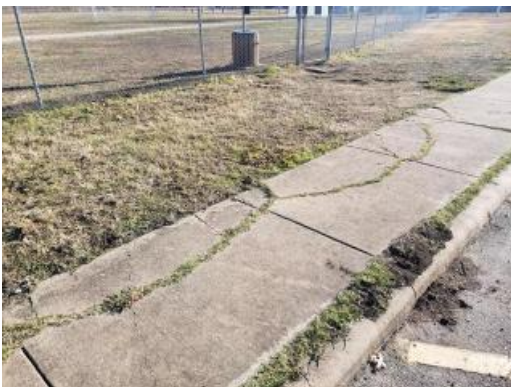
Cracked concrete sidewalk
