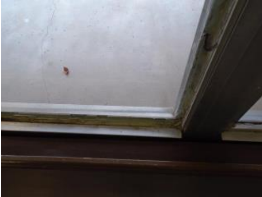
Damaged window frame
