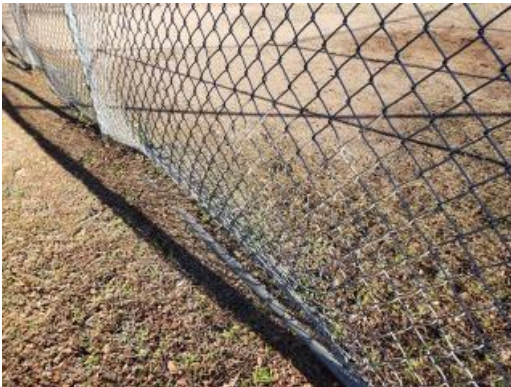
Damaged chain link fence
