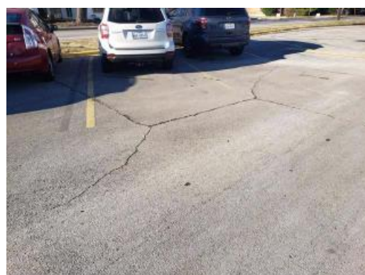
Cracked asphalt paving
