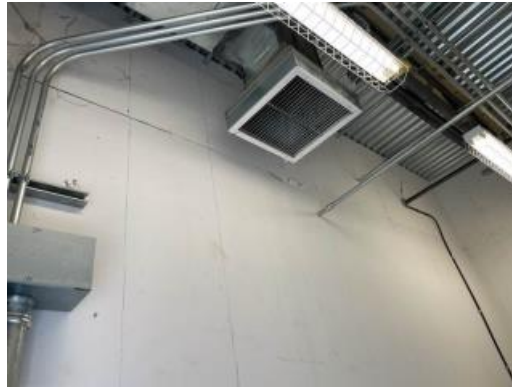
Interior walls in need of paint
