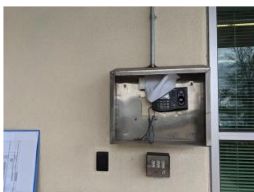
Damaged Entry Code
