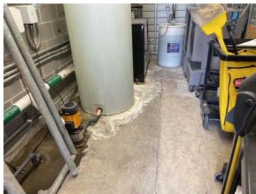
Bus washing flooring needs power wash
