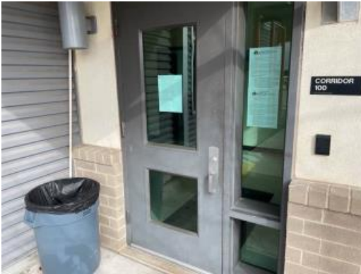
Exterior doors are fading
