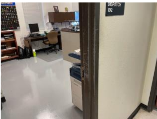
Interior door frames to be repainted
