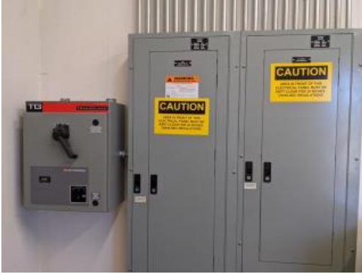
Typical Electrical Panels
