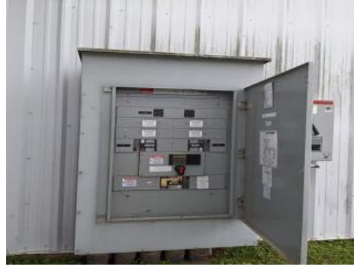
Exterior Mounted Electrical
