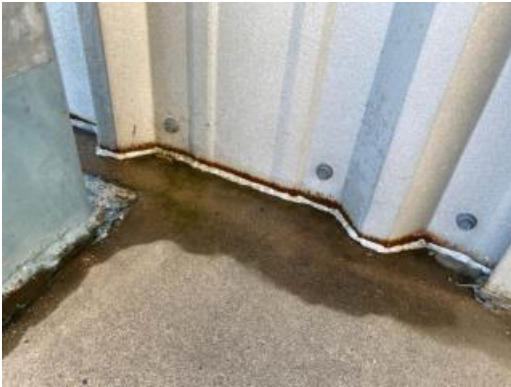
Rusted base of metal panel
