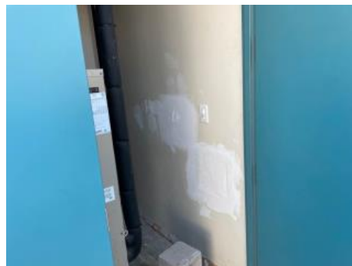
Wall to be repaired and repainted
