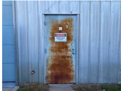
Rusted steel door
