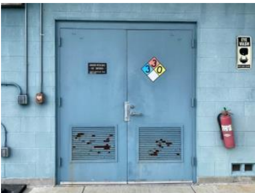
Rusted and sun bleached steel doors
