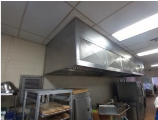
Kitchen exhaust hood
