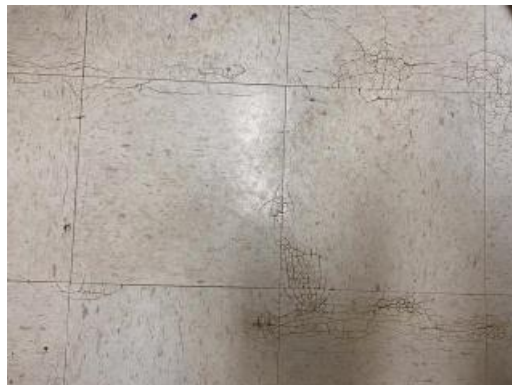
Vinyl composite tile needs replacement
