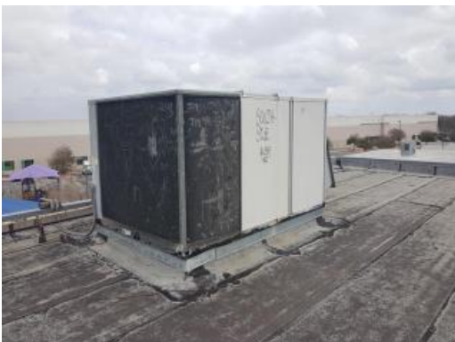
RTU reaching the end of its useful life
