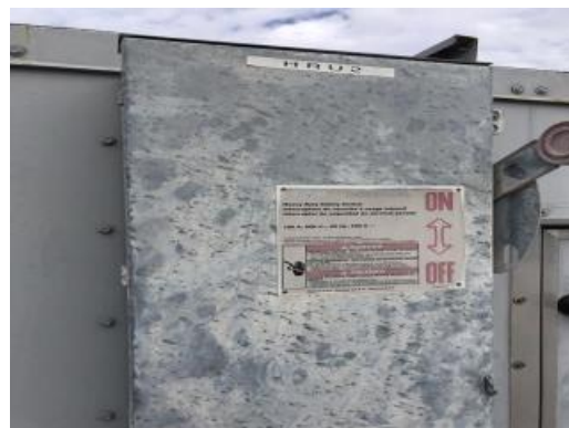
Electrical panel is well worn
