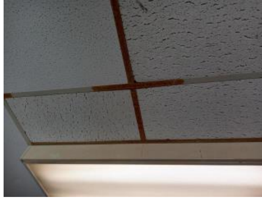
Outdated acoustical ceiling tiles and grid
