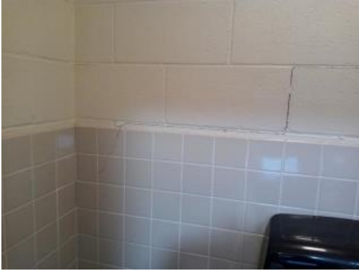
Ceramic tile is cracked
