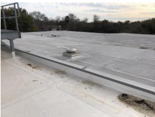
Roof and exhaust present wear
