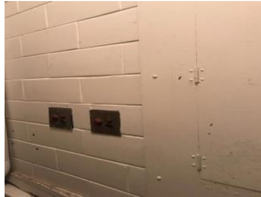
Interior wall presents wear
