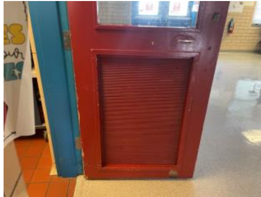
Kitchen access wood door near end of life.
