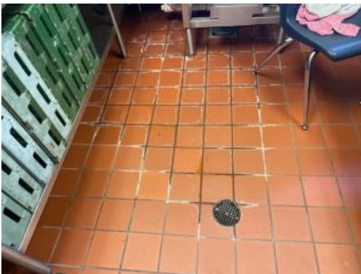
Kitchen tiles at end of life
