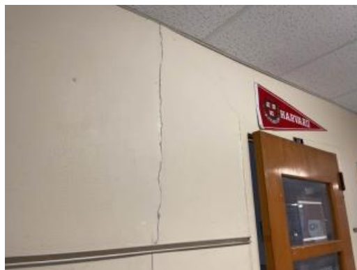
Cracked interior walls
