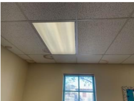
Water stains and sagging grid in classroom acoustic ceiling tiles
