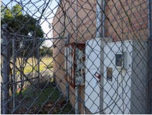
Building electrical service is beyond its useful life
