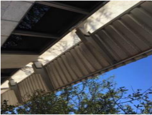
Awning steel rusting
