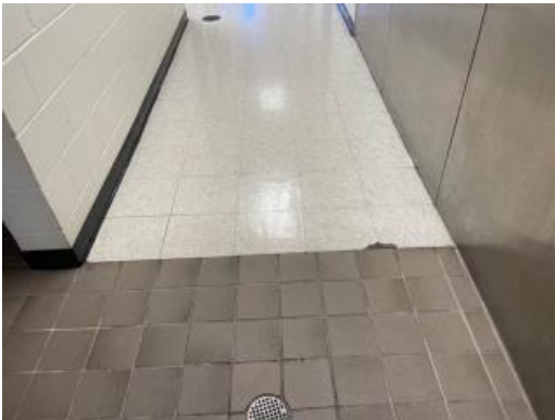
Damaged vinyl composite tiles
