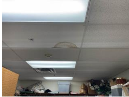
Stained ceiling tiles
