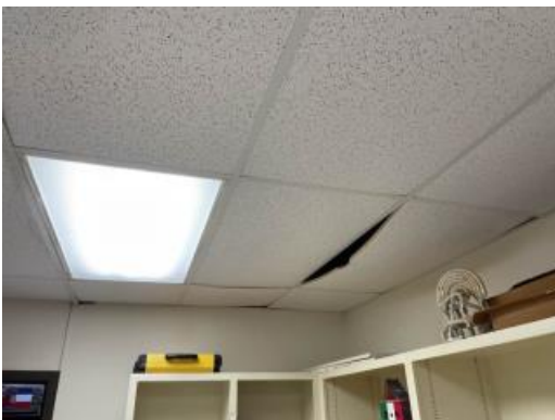
Warped ceiling tiles
