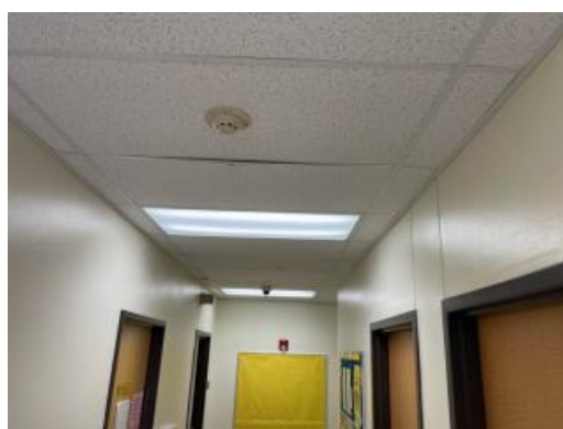
COR7- Acoustic ceiling grid sagging along with chipped tiles.
