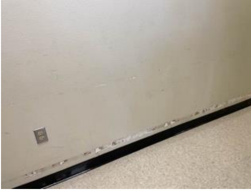
Walls painting peeling
