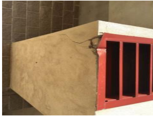
Damaged stucco, southeast corner.
