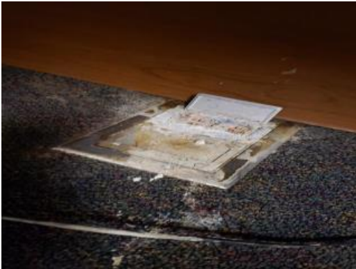
Corroded floor electrical box
