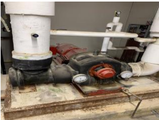
Corroding pumps and rusting area
