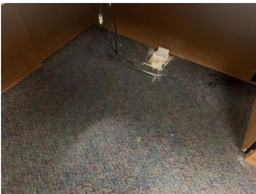
Exposed electrical equipment
