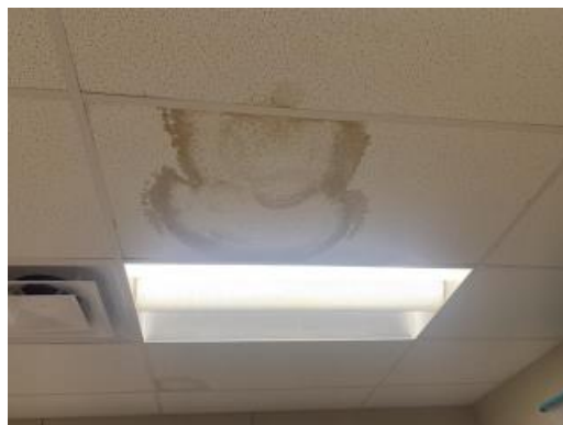
Stained acoustical ceiling tiles
