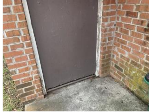
Metal Door chipped at bottom
