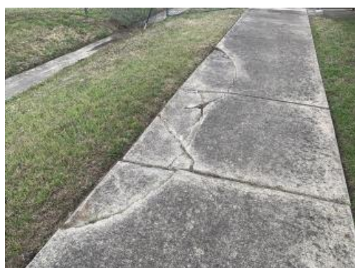
Sidewalks are worn
