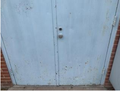
Metal Doors are rusted
