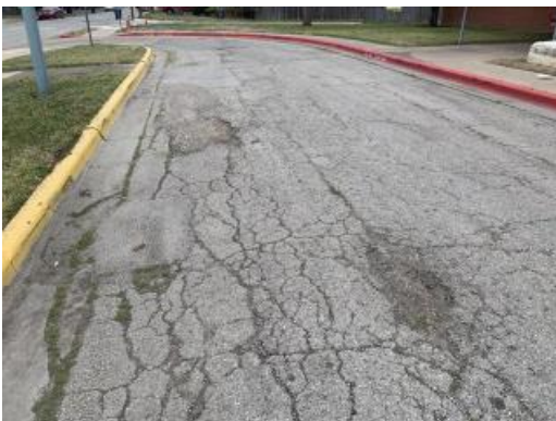
Asphalt Drive shows wear
