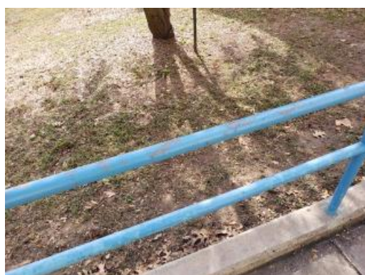
Rusted metal handrail
