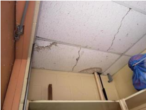
Broken acoustical ceiling tile
