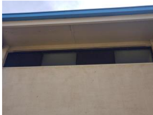
Damaged exterior insulation finishing system
