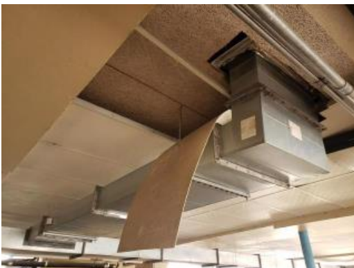
Damaged vinyl ceiling
