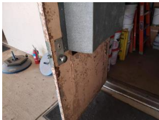
Damaged exterior metal door
