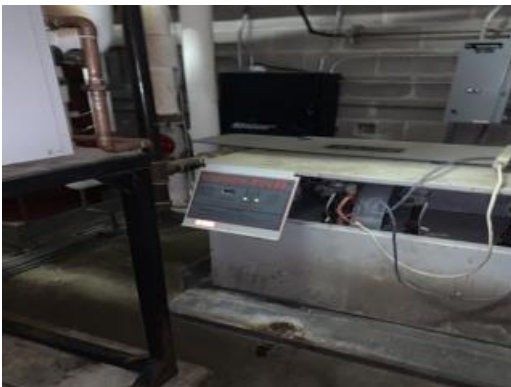
Exposed wiring in mechanical Room
