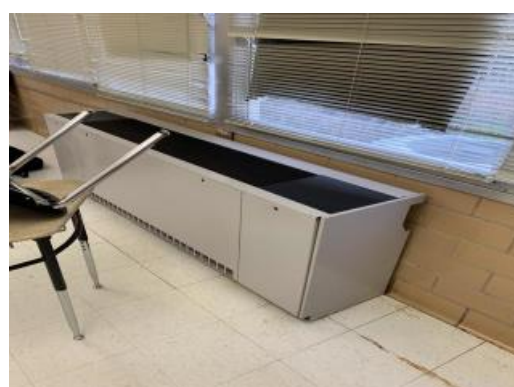
Aged ventilation Unit
