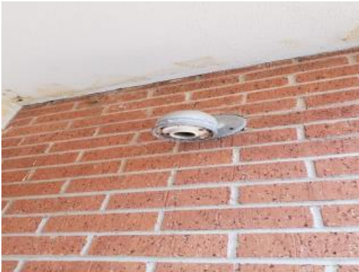
Missing light fixture
