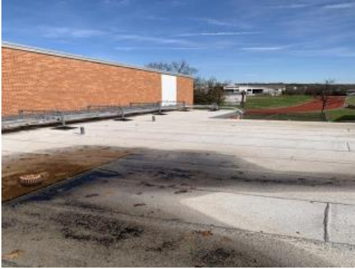
Water pooling will eventually cause serious damage
