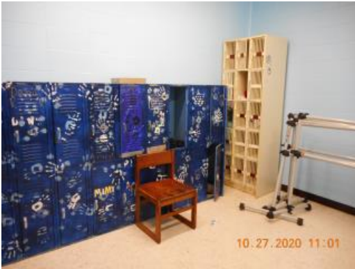
Damaged and broken lockers
