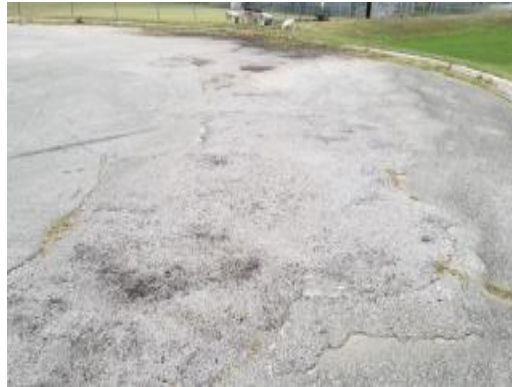
Broken asphalt pavement
