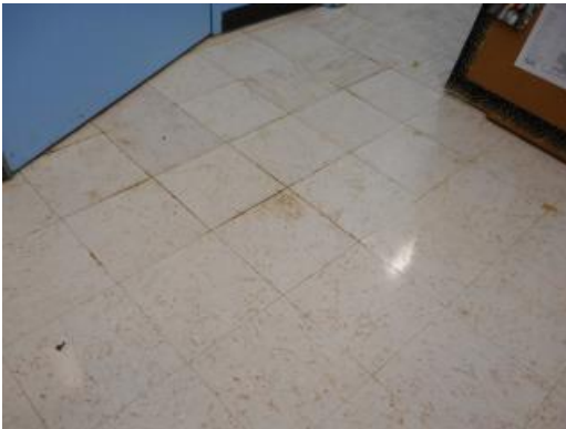
Damaged vinyl composition tiles
