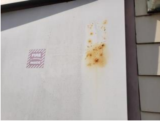
Rusted exterior door
