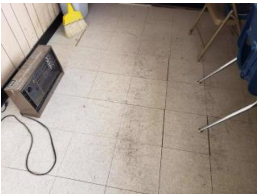
Damaged vinyl composition tiles
