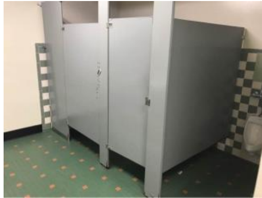
Restroom partitions rusted and damaged
