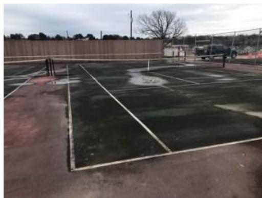
Site tennis courts beyond service life
