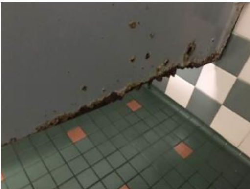
Restroom partitions rusted and damaged
