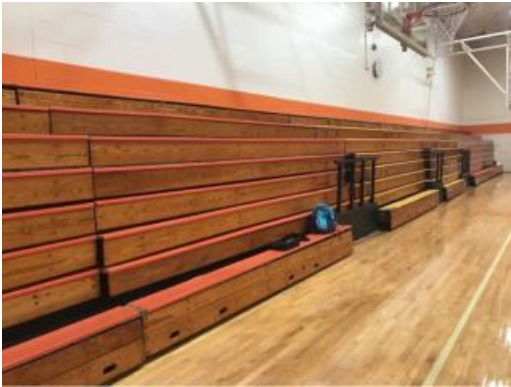
Gym bleachers beyond service life and reported safety issues
