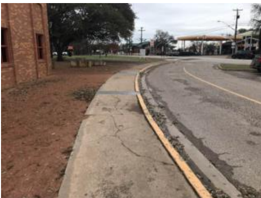
Site sidewalk damage south side
