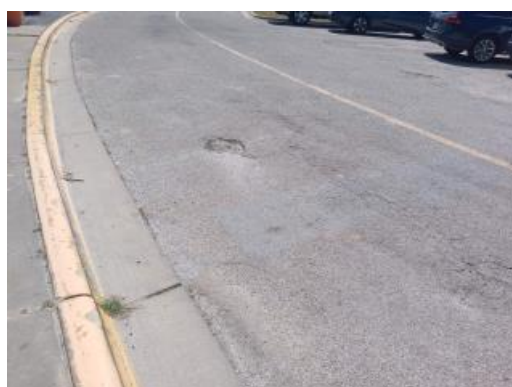
Pavement is cracked
