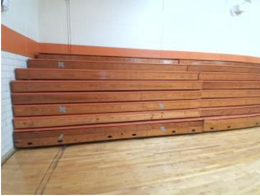
Gym seating is worn
