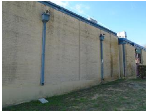
Exterior wall is stained
