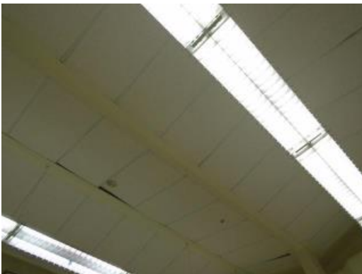
Acoustical ceiling tile (ACT) bowing and warped
