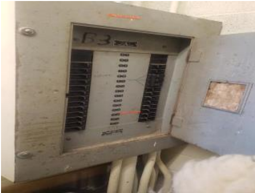
Dated electrical distribution panels
