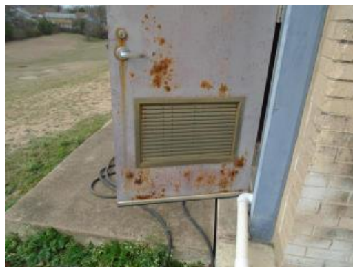
Corroded metal door
