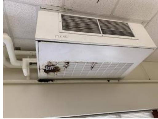
Aged unit ventilator
