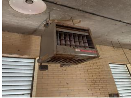
Electric unit heaters are beyond their useful life
