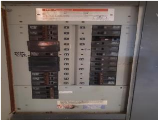
Electric distribution panel beyond its useful life
