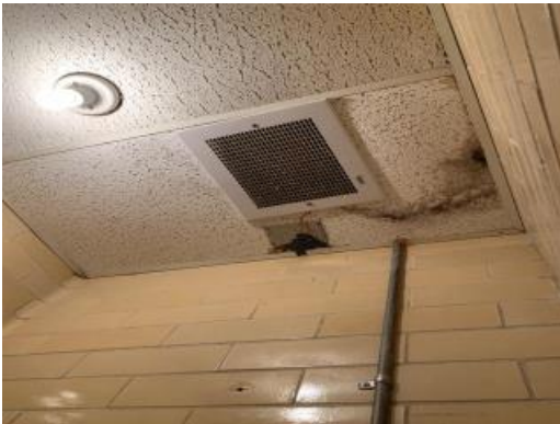
Ceiling tile is damaged
