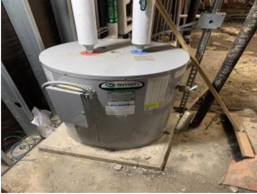
Water heaters are reaching the end of their useful life
