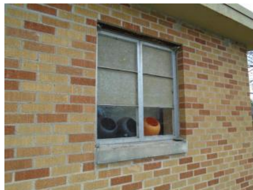
Exterior aluminum windows are past useful life
