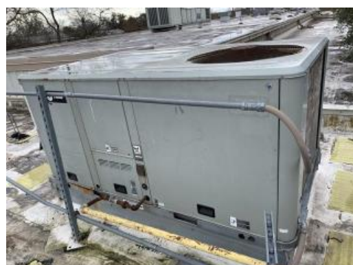
Roof top unit is aged
