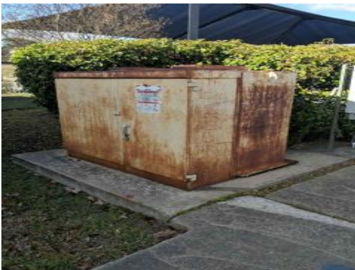
Rusted transformer on northwest side
