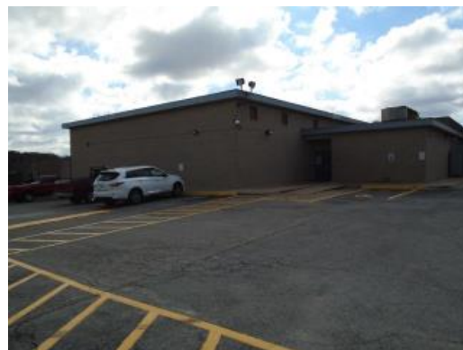
Cracked parking lot asphalt pavement
