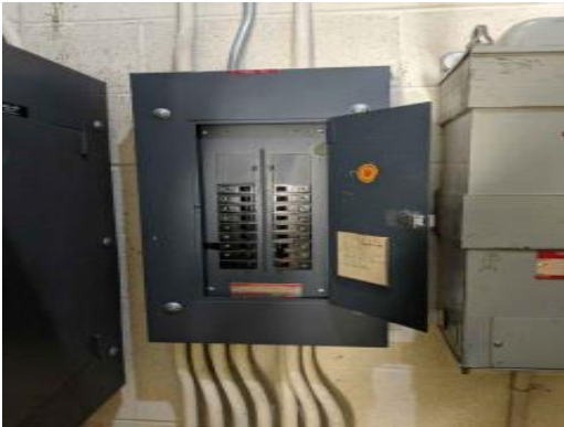
Electrical panel at end of life
