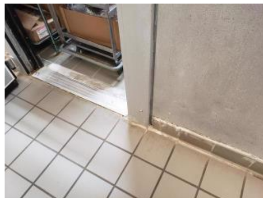
Over caulking on tile baseboards
