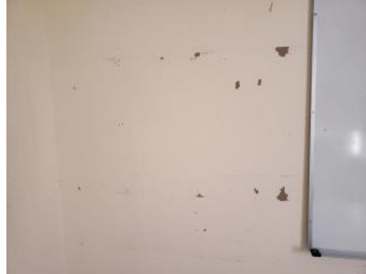
Wall finishes present scuffing
