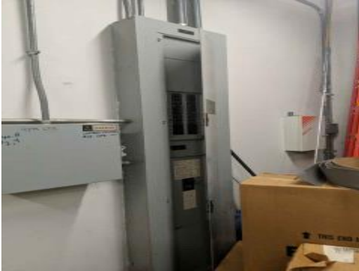
Electric Panel is hard to reach
