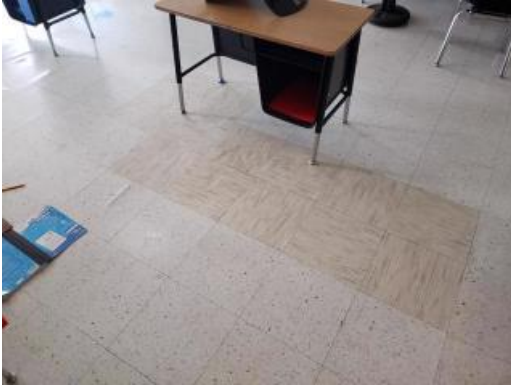
Vinyl composite tile flooring is patched and at the end of its useful life.
