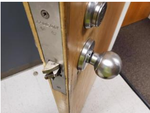
Door hardware is not accessible
