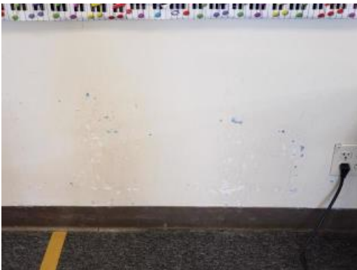
Wall is worn and aged
