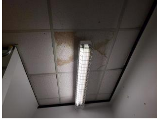
Stained ceiling tiles.
