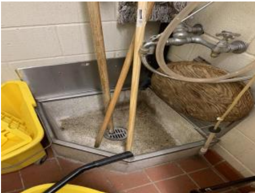
Mop sink is beyond service life.
