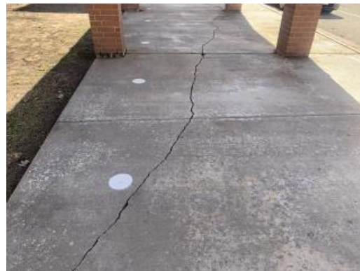
Cracking in concrete walkways.
