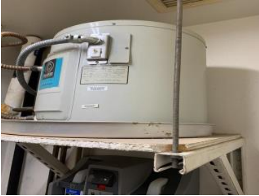
Electric water heater is supported by shelf.
