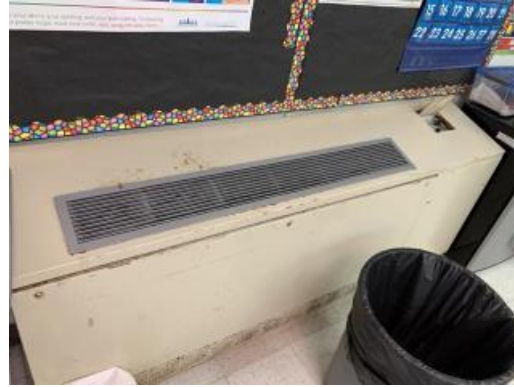
Unit ventilator is beyond service life.
