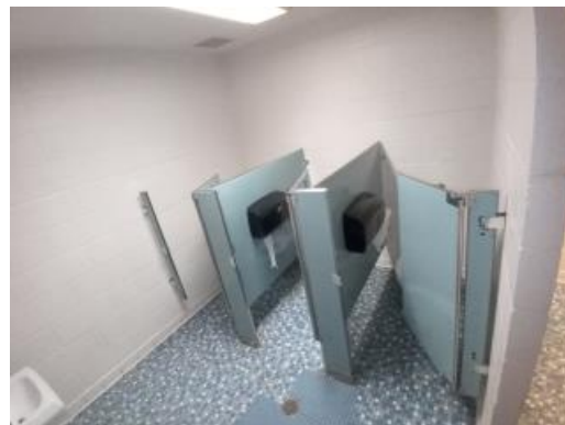
Well worn toilet partitions
