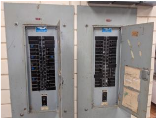
Outdated Electric panels
