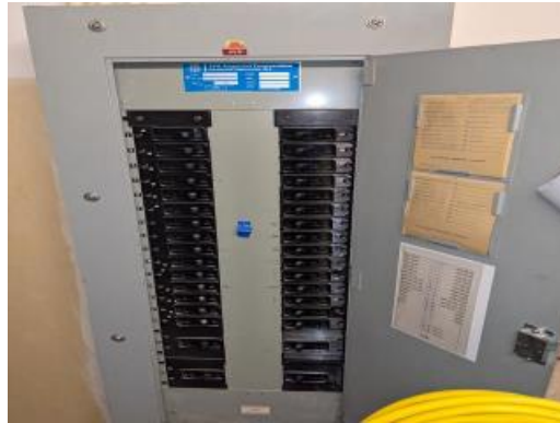
Typical Electrical Panel
