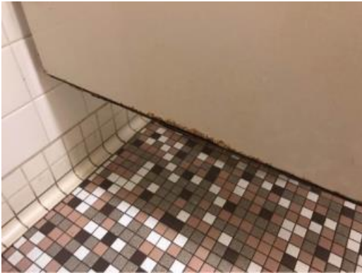
Student restroom partitions are rusted and beyond service life.
