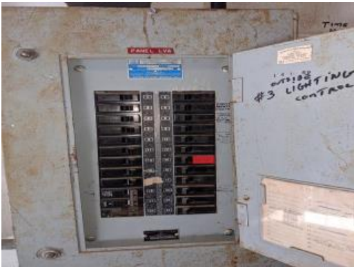
Distribution panel is aged and rusted.
