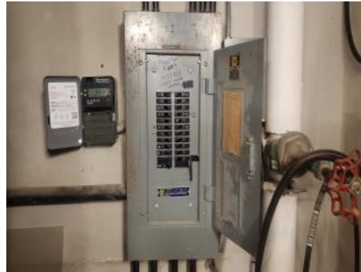
Typical Electrical Panel
