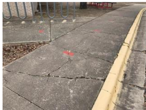
Concrete sidewalk has numerous cracks.
