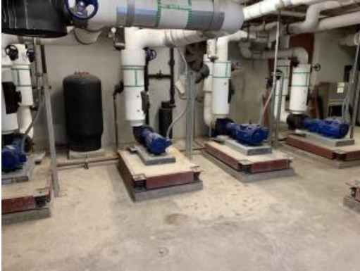
Chilled water pumps
