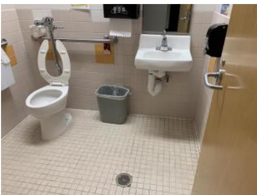
Typical plumbing fixtures
