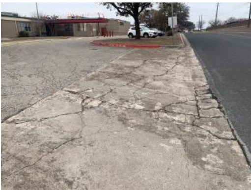
Concrete drive has numerous cracks.
