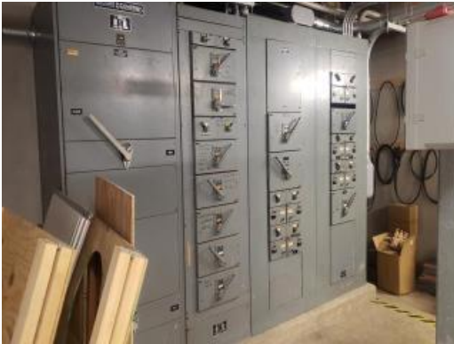
Main Switch gears
