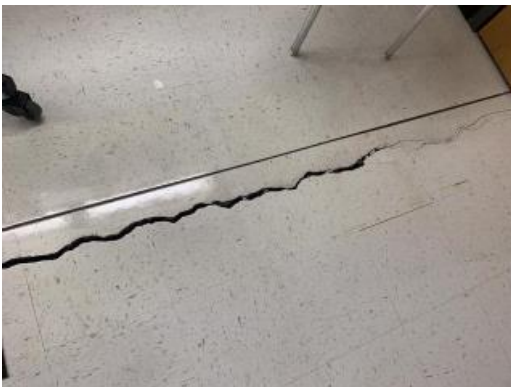
Damaged vinyl composition tile floor
