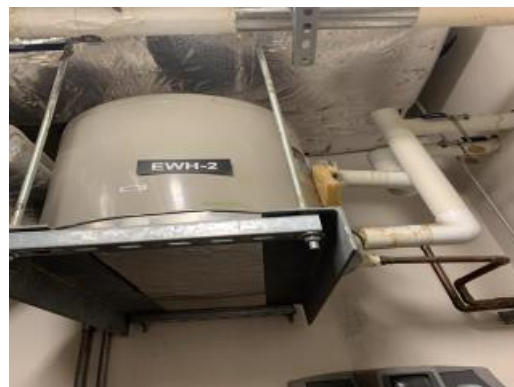
Water heater beyond useful life
