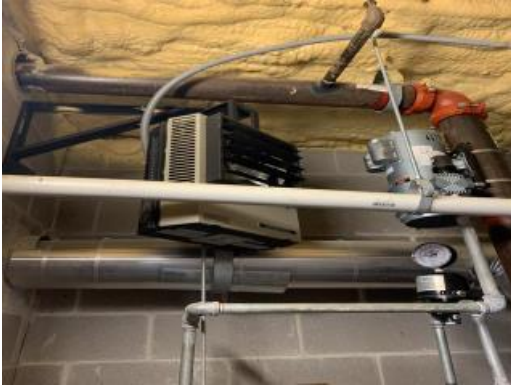
Unit heaters beyond useful life
