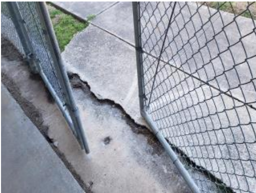
Crack in pavement
