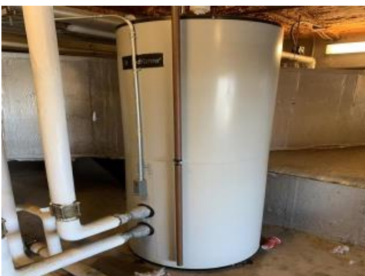
Water heater past expected life
