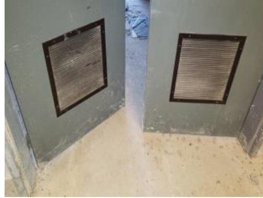
doors are damaged and worn
