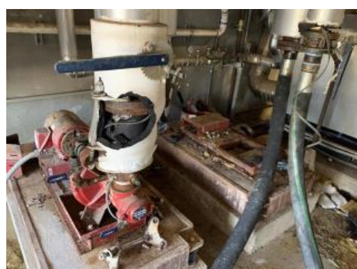
Pumps beyond useful life
