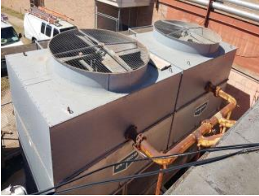
Cooling tower rusted
