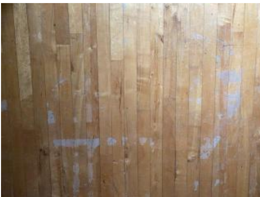
Wood floor worn and stained
