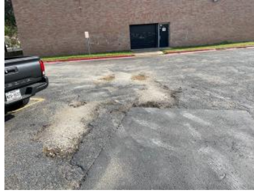
Damaged asphalt in parking lot
