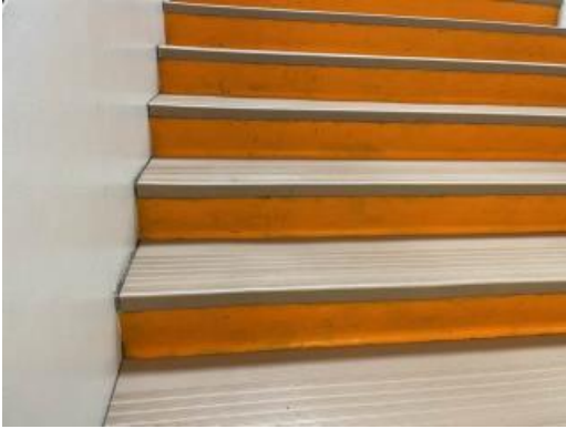
Rubber stairs are worn and torn
