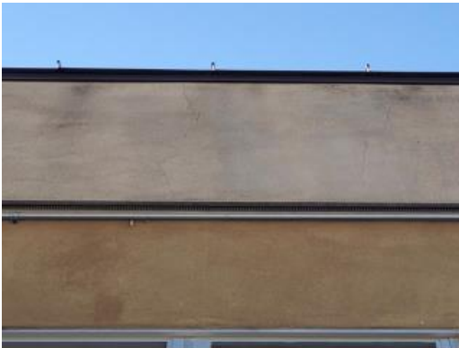
Aged exterior walls
