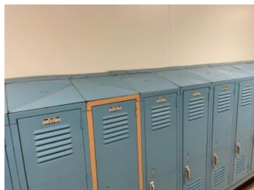
Hallway lockers beyond useful life
