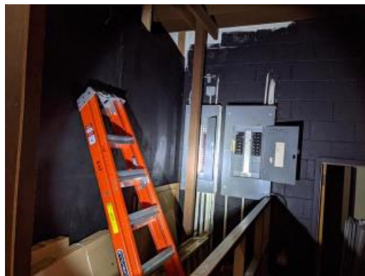
Obstructed electrical panels
