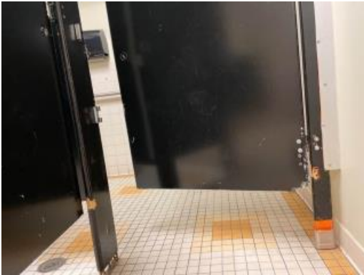
Restroom partition walls past useful life
