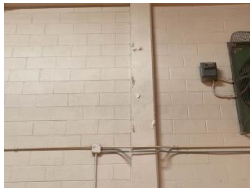
Gym wall paint is beyond useful life
