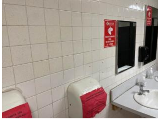
Restrooms wall tiles past useful life
