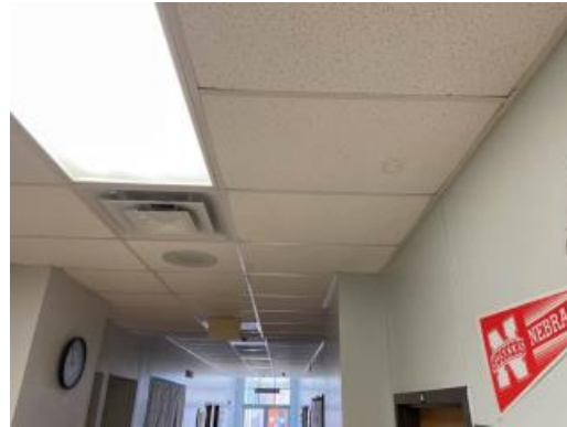
Stained and sagging acoustic ceiling system
