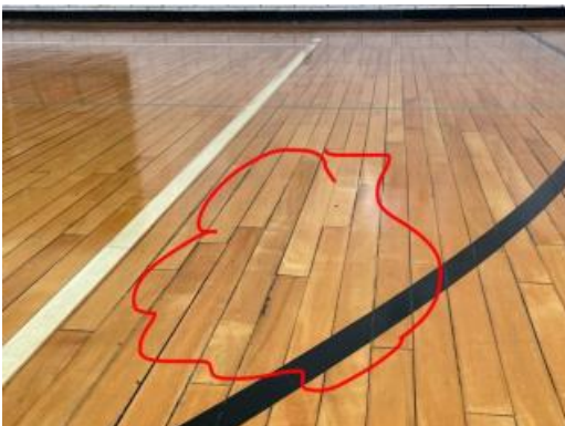
Buckling wood floors
