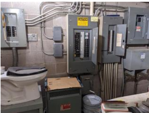
Electrical panels are past useful life
