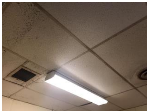
Aged ceiling tiles
