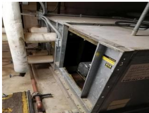
Aged mechanical equipment
