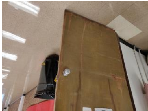
Deteriorated wood door
