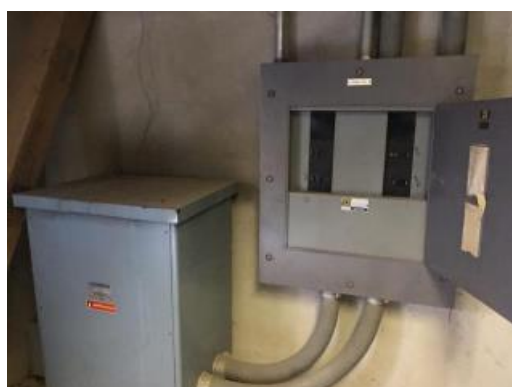
Electrical Panels and Transformer
