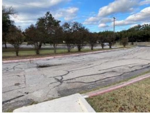
Aged asphalt pavement
