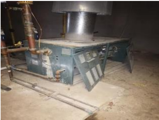
Aged mechanical equipment
