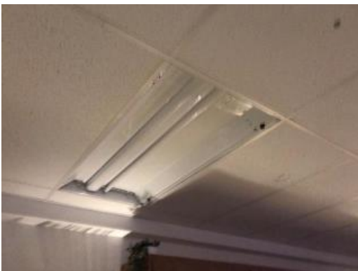
Damaged light fixtures
