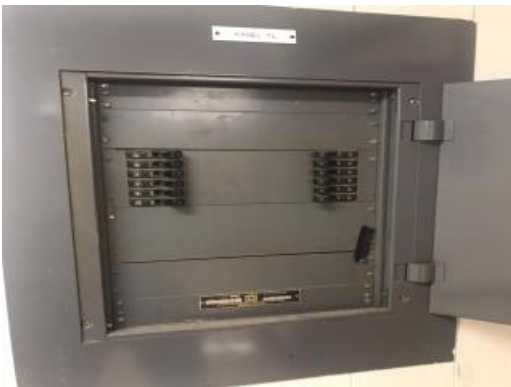
Aged electrical distribution panels
