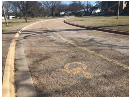
Asphalt drive past useful life
