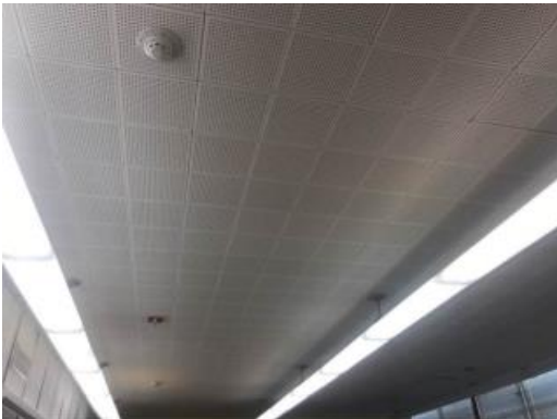
Deficient ceiling tiles
