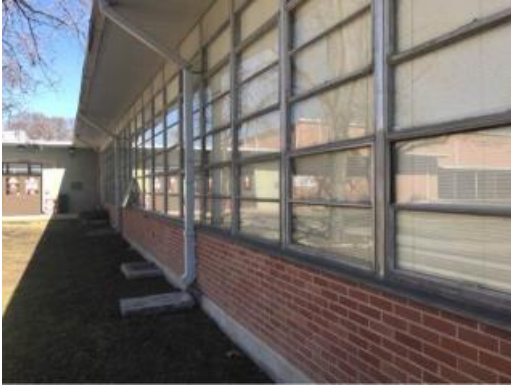
Exterior windows beyond service life
