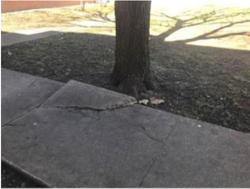
Concrete sidewalk damage
