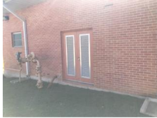
Exterior door deficiency
