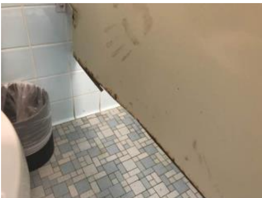
Aged toilet partitions
