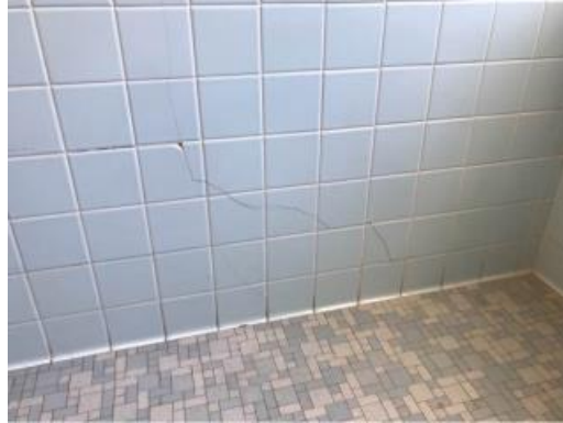
Damaged ceramic tiles
