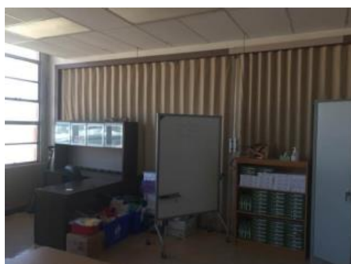
Deficient folding wall panels
