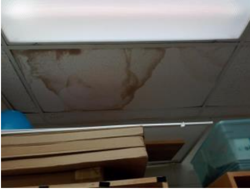
Stained ceiling tiles
