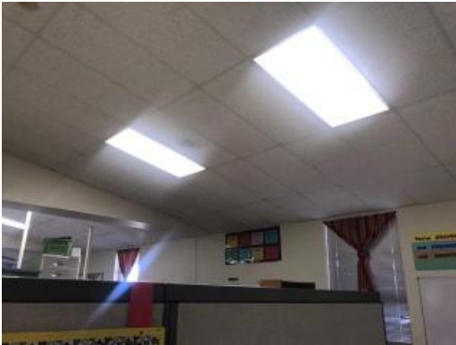
Aged acoustical ceiling tile
