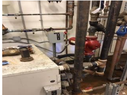
Aged boiler and heating water pipes
