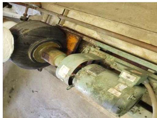
Corroded chilled water pump
