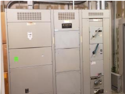
Main Switch Gear
