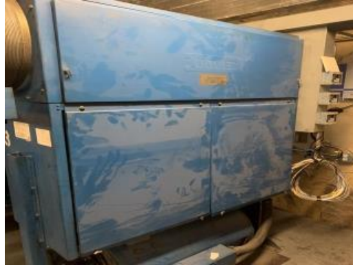
Typical AHU equipment
