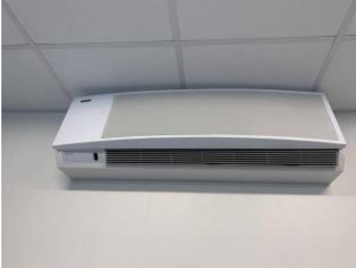
Air conditioning unit
