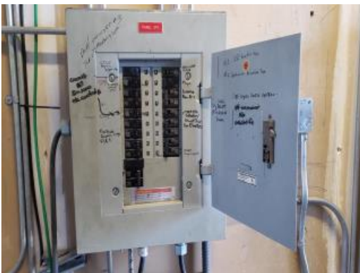
Aged Electrical Panel
