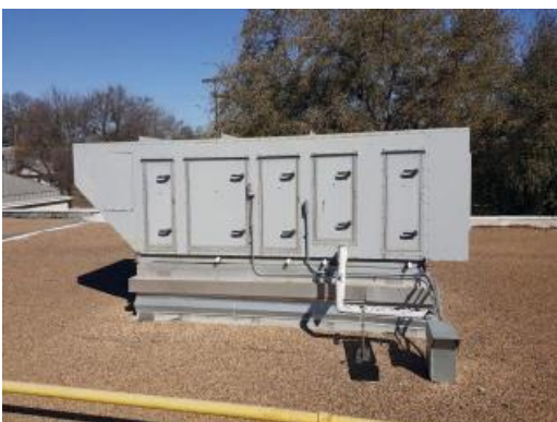
Roof Top Unit
