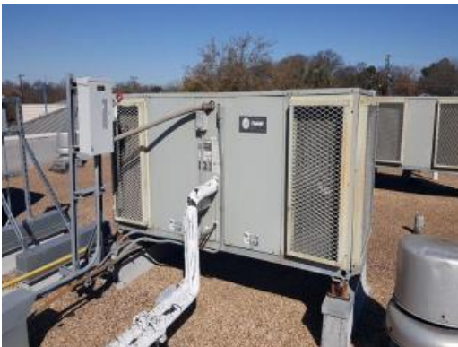
Roof Top Unit
