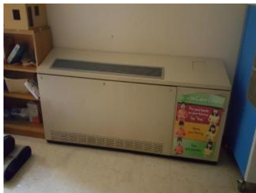
Aged air conditioning unit
