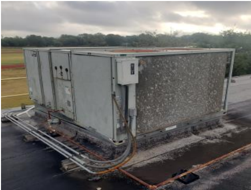
Condensing unit reaching end of life
