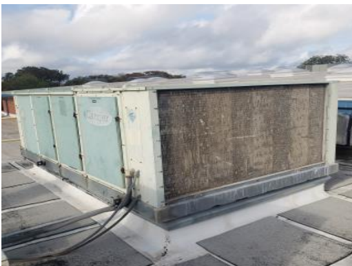
Roof top unit is beyond its useful life
