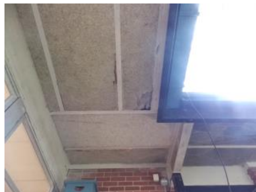
The soffit is damaged
