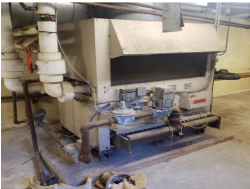
The basement boiler is beyond its useful life
