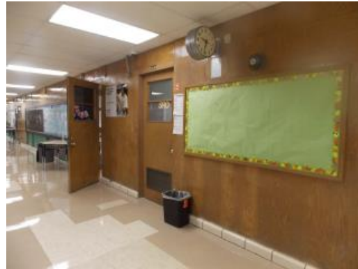
Worn wood panel and door
