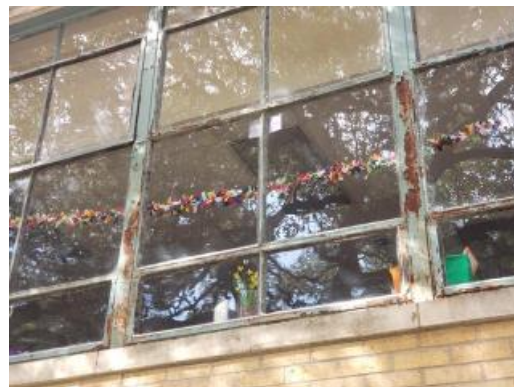
Exterior windows are beyond their useful life
