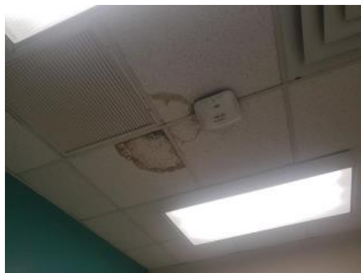
Stained ceiling tiles
