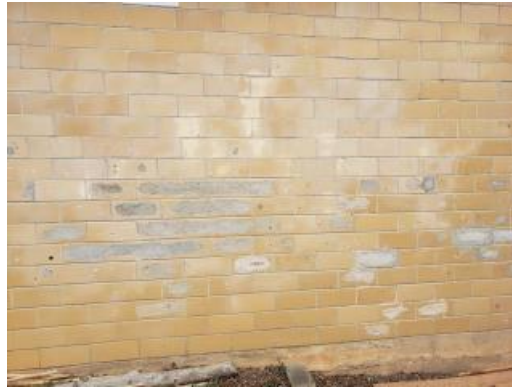
Exterior wall damage
