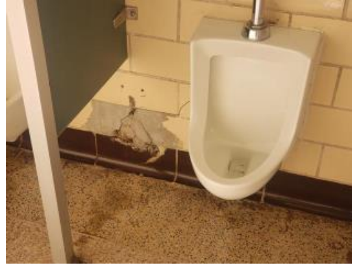
Aged plumbing fixtures
