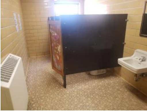
Aged toilet partitions
