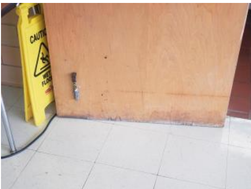
Interior wood doors show signs of wear
