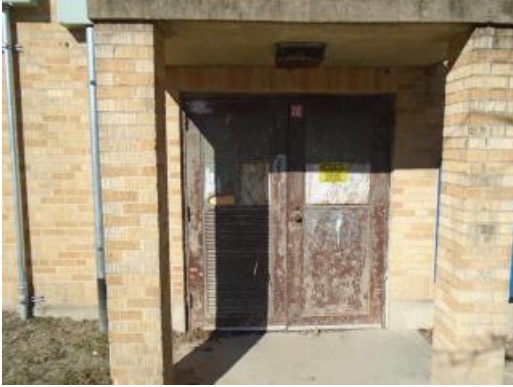
Exterior doors beyond useful life
