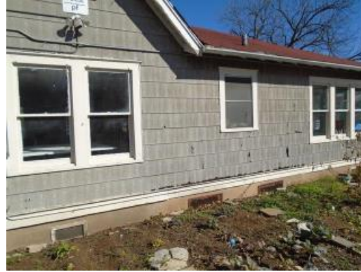
Exterior windows are beyond their useful life
