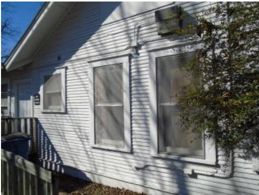
Exterior Windows are beyond their useful life
