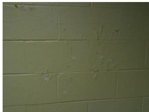
Peeling wall paint
