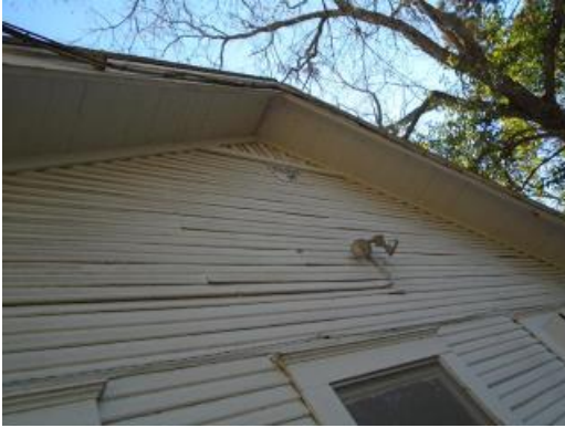
Exterior wood siding is at the end of its useful life
