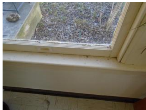
The exterior windows are beyond their useful life.
