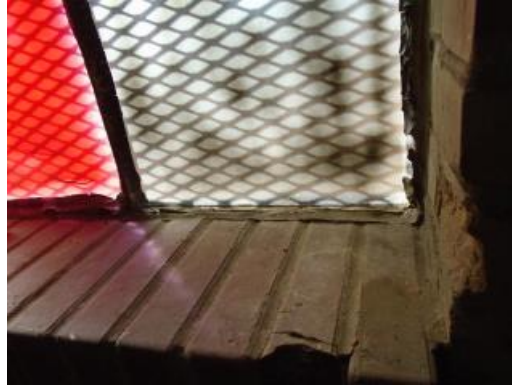
Windows at the mechanical building are beyond their useful life
