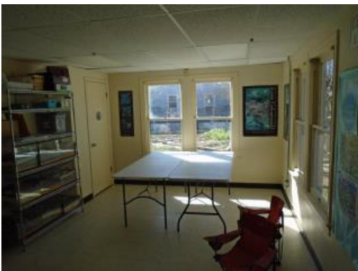
Interior finishes are worn and outdated.
