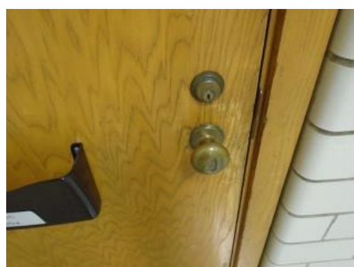
Outdated door hardware
