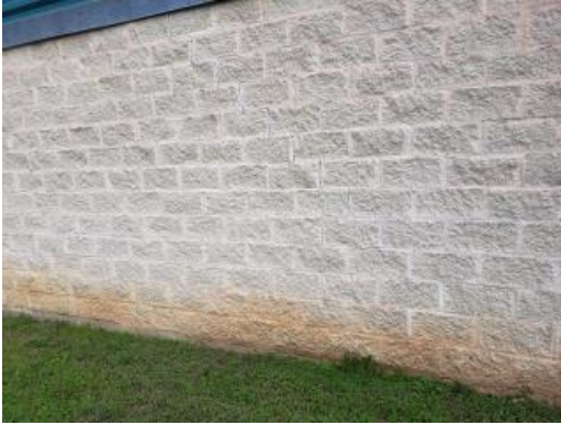
Exterior walls stained
