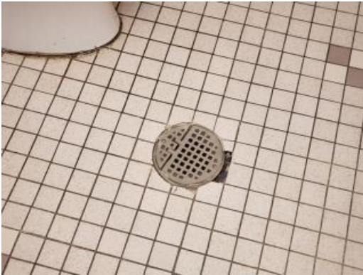
Damaged and old ceramic tile floors
