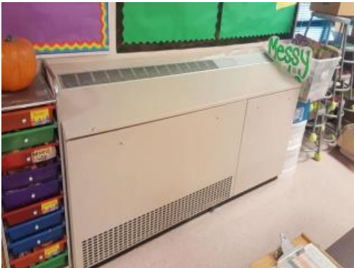
Outdated unit ventilator in classrooms
