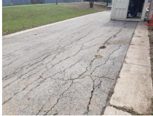
Cracked asphalt pavement
