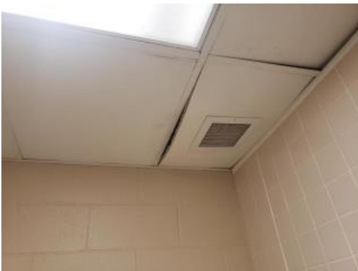
Sagging ceiling tiles
