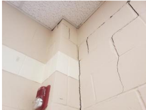
Possible foundation settlement
