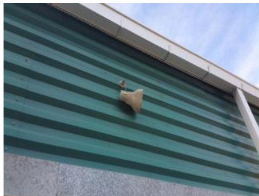
Broken exterior lighting
