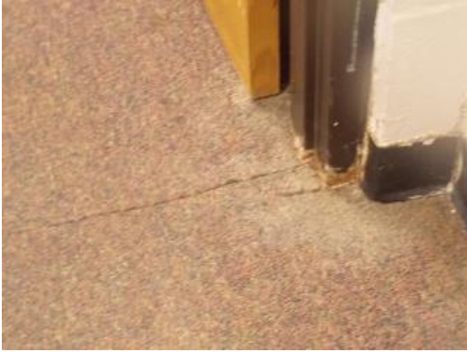
Interior doorway damage
