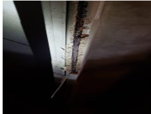
Exposed rebar in basement
