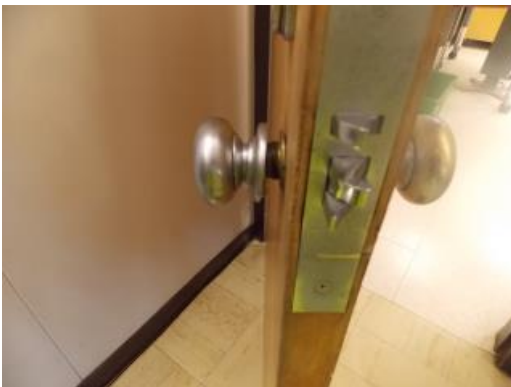
Damaged door hardware
