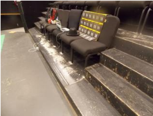
Worn theater flooring
