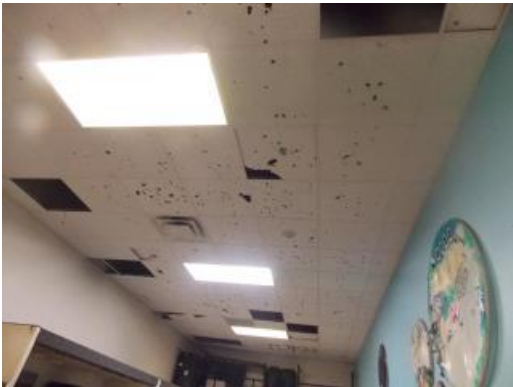
Aged ceiling tiles
