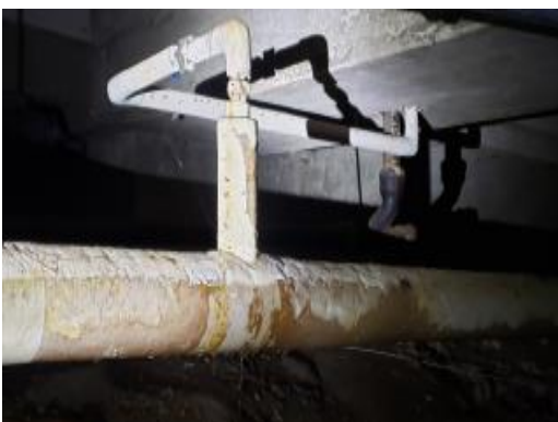
Pipes leaking in crawl space
