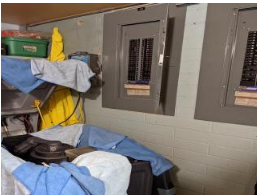
Obstructed electrical panel
