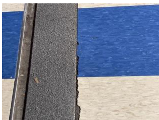
Chipped and worn ceramic tile flooring.
