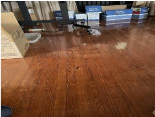
Scratched and worn wood floor panels.
