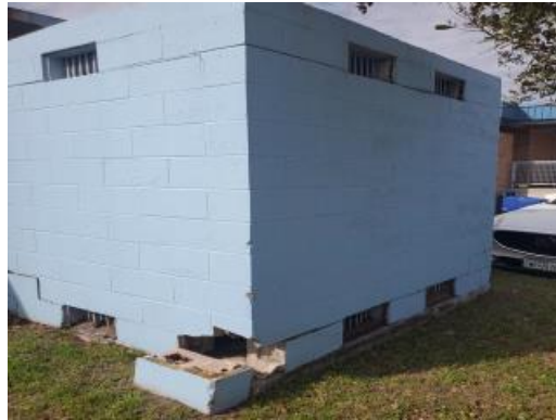
Damaged building exterior
