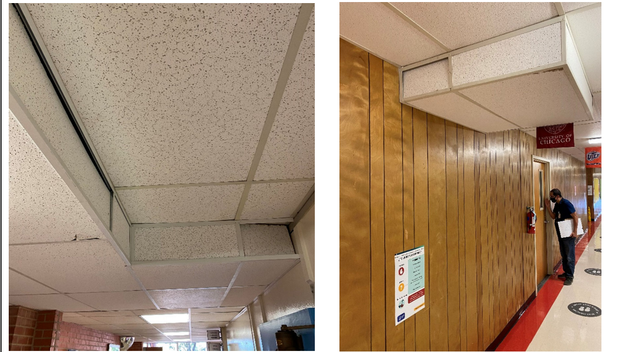
Ceilings are low and in aged condition. Signage and clocks mounted as close to ceiling as possible.
