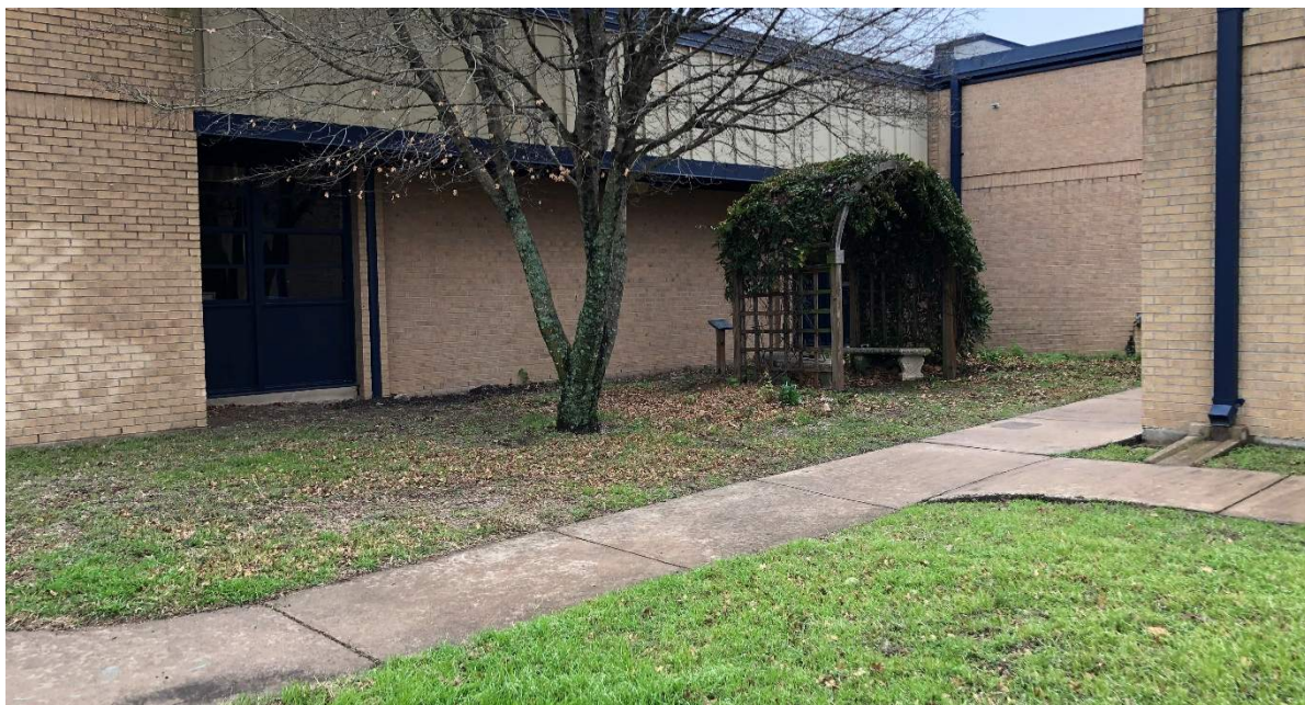
Small outdoor learning space with insufficient seating and needs further development.
