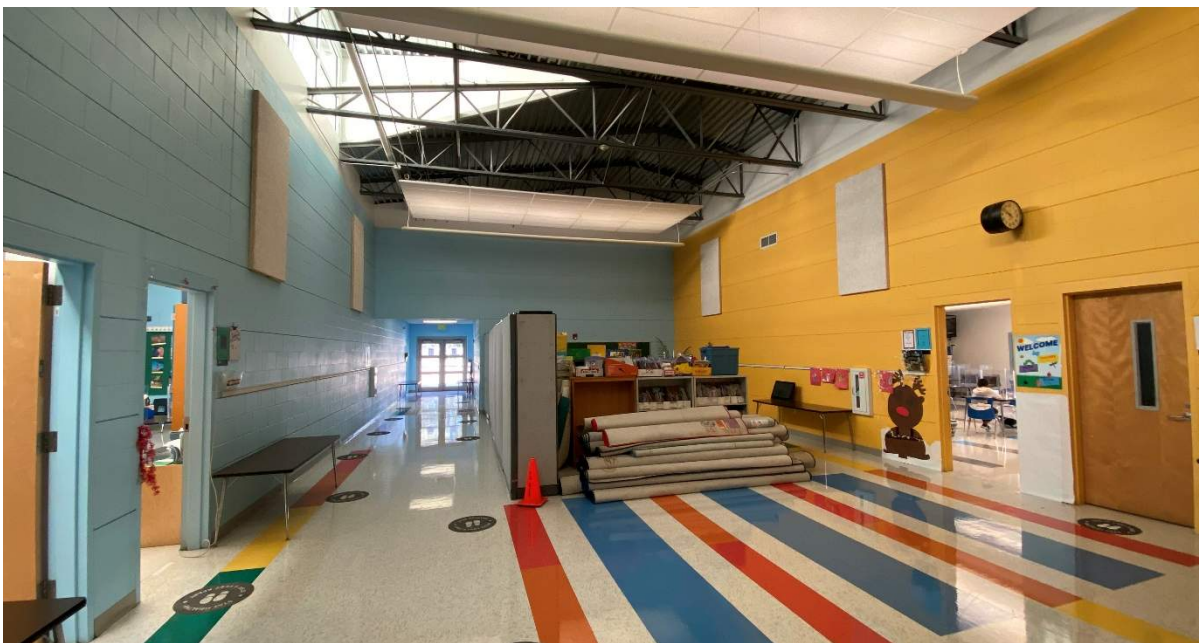
Academics and Learning: Breakout space between studios used as storage. Storage appears to be an issue. This could be an outcome of COVID-19 protocols and does not necessarily reflect a normal school year.
