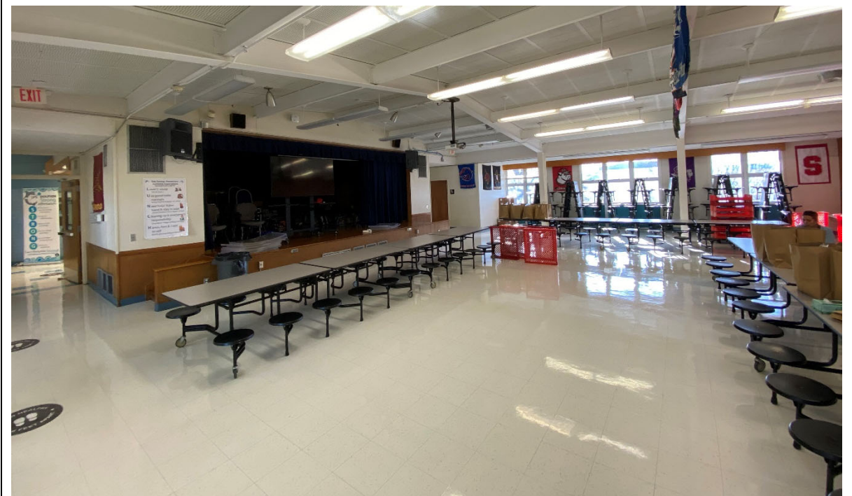
Cafeteria stage is not ADA accessible, and storage is inadequate. There is no variety in the types of seating provided.
