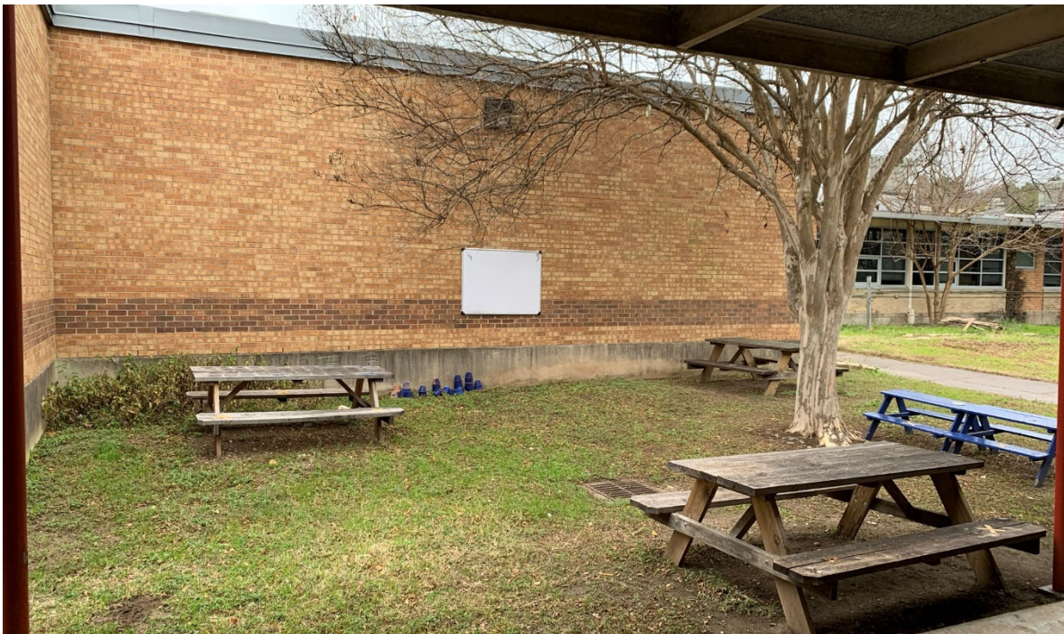
The courtyards throughout campus are well used due to their close connection to each studio wing, as each room opens to the exterior. Furniture needs updates.
