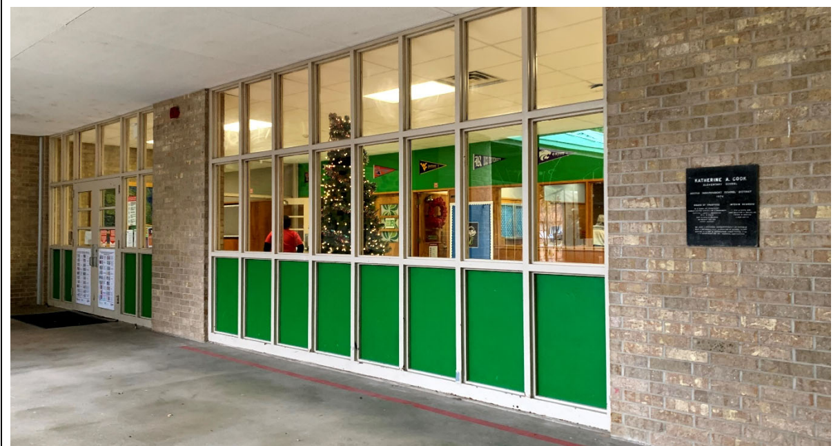
Front entry door has limited glass. There is no secure vestibule. Main office is at front entry and has limited line of sight to the front door.
