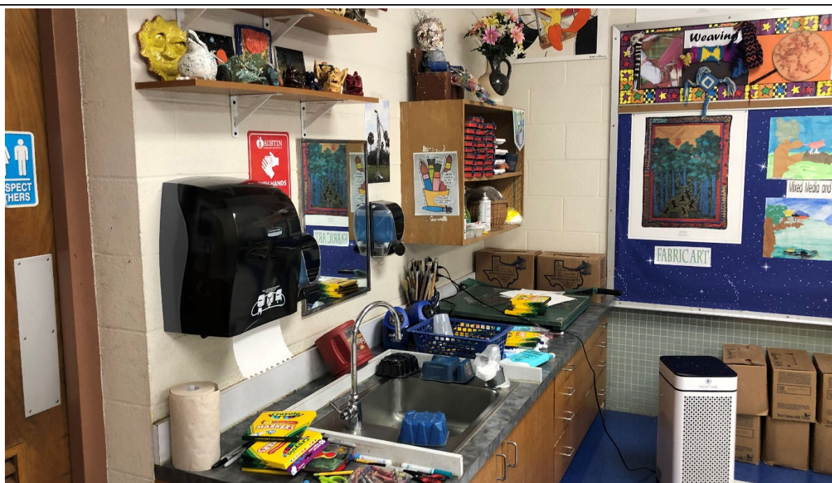
Sink in art room is insufficient for function of art room.
