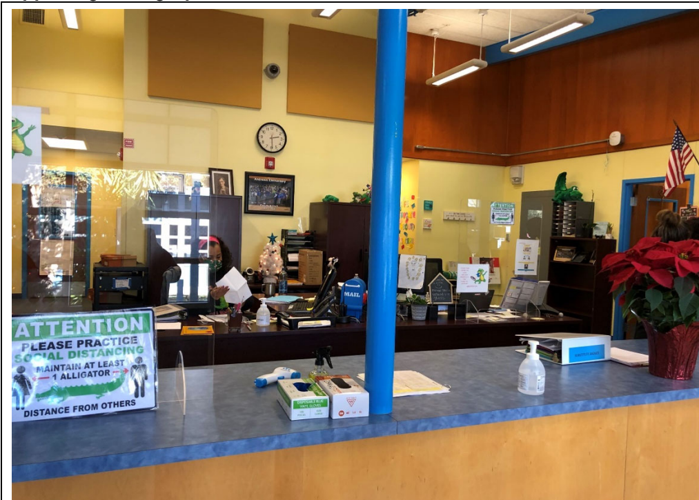
Administration Spaces: Reception is adequately sized and feels welcoming, but finishes need updates.
