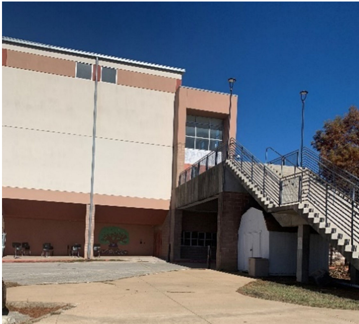
No covered walkway at bus drop-off.
