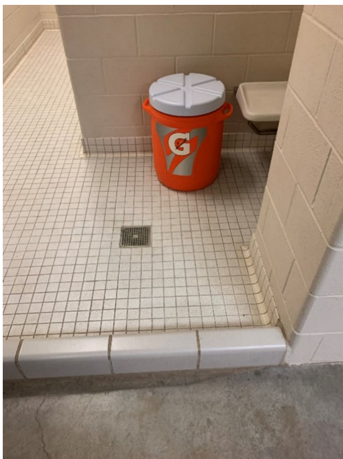
Locker rooms in athletics/fitness department has ADA issues at shower areas.
