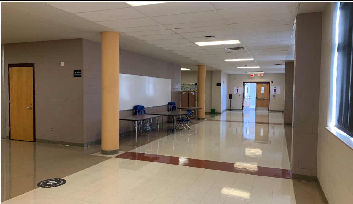
Main corridors are large and open with lots of daylighting and are in good condition.
