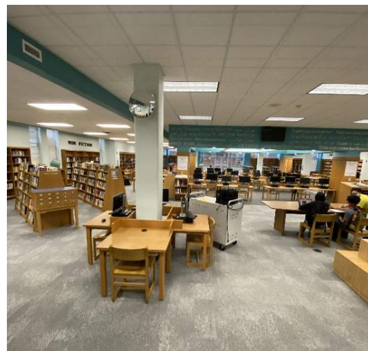
Media Resources: Library is in good condition and is adequately sized. Furniture throughout is dated and heavy (though in decent condition). More power/data is needed as messy power strips and cords cause clutter.
