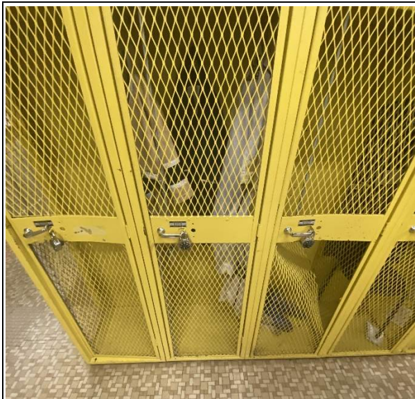
Athletics lockers throughout are dated – products and their parts have been discontinued, so maintenance is nearly impossible.
