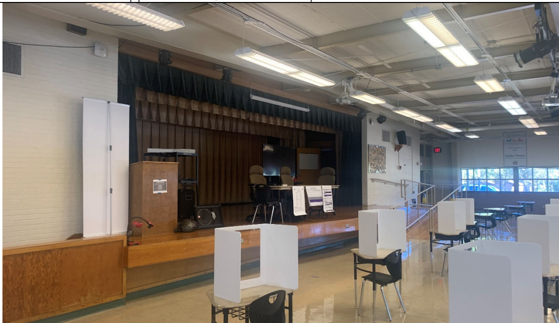
Cafeteria stage: A/V equipment/stage condition is unsatisfactory and difficult to use for productions and meetings.
