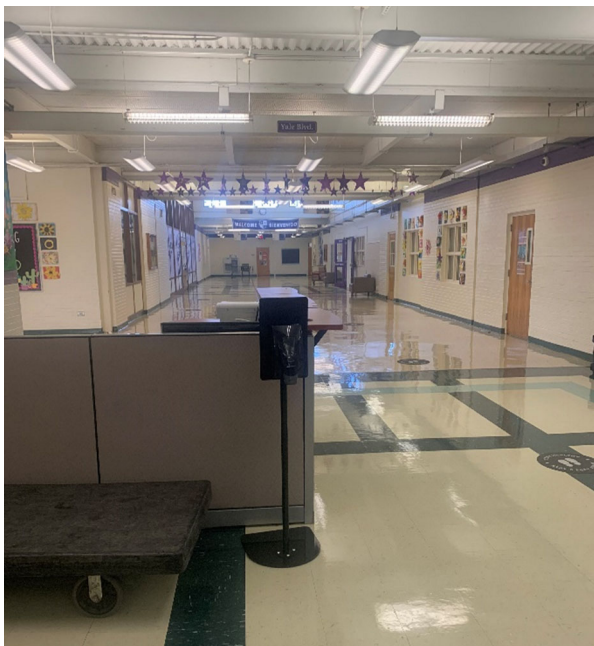
Main entry: [REDACTED] Main corridor is generous in width and could support informal/collaboration spaces.
