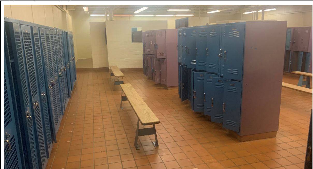
Locker rooms: Dated finishes and there are accessibility issues.
