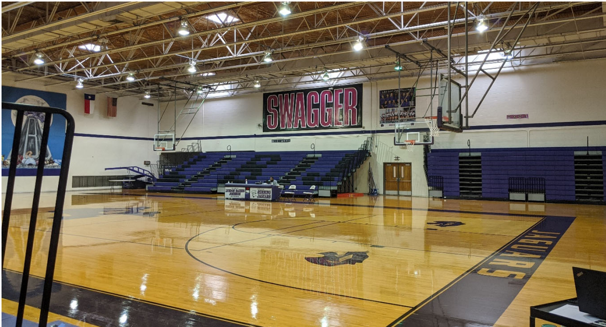
Gym is original to school. Insulation falls from exposed ceiling and paint is peeling from walls.
