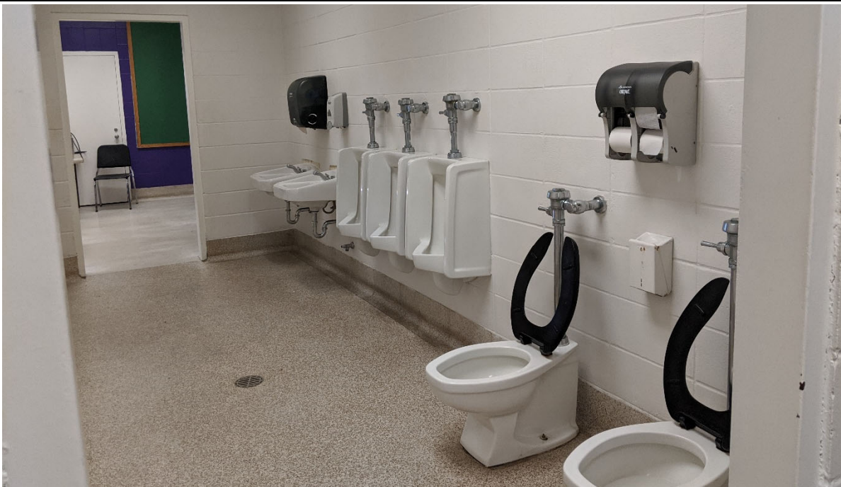
Locker rooms are in poor condition and lack privacy.
